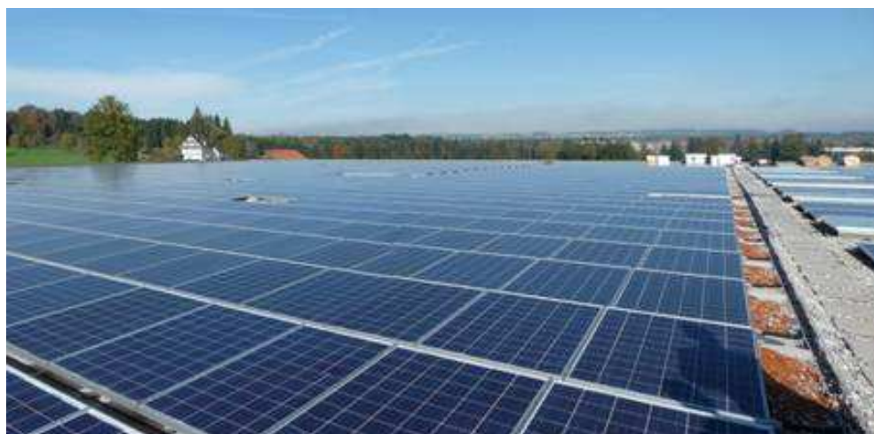
View of part of the facility on the flat roof of the new goods depot. The recumbent array of the modules was dictated by the maximum allowable building height. Pistor-Edisun Power solar power facility
