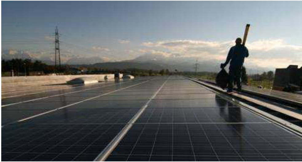
View of the facility atop the factory building upon completion of construction. The two halves of the roof have been covered in modules. Pistor-Edisun Power solar power facility
